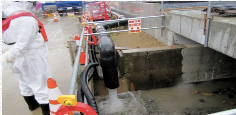
Tank leaks 300 tons of radioactive water at Fukushima plant, The Asahi Shimbun, August 20, 2013,
